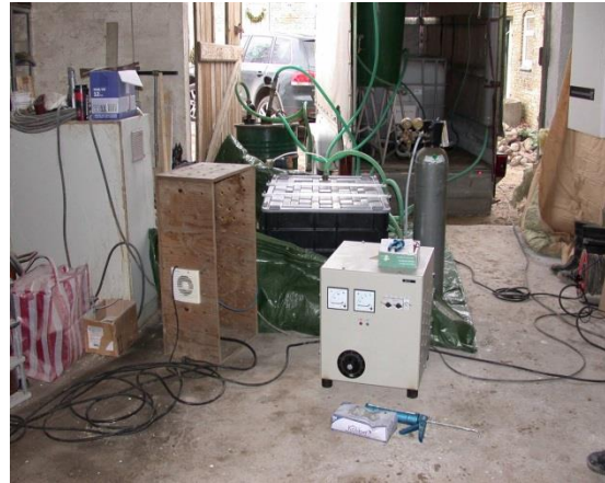
Fig. 2: Converter (grey), reactor, CO 2 bottle, on trailer: tank, stripping reactor and filter.
